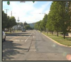
Roadway with Poor Pavement SR 1025 in Berwick Borough, Columbia County
