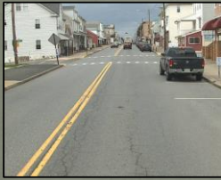
Roadway with Poor Pavement SR 61 in Kulpmont Borough, Northumberland County
