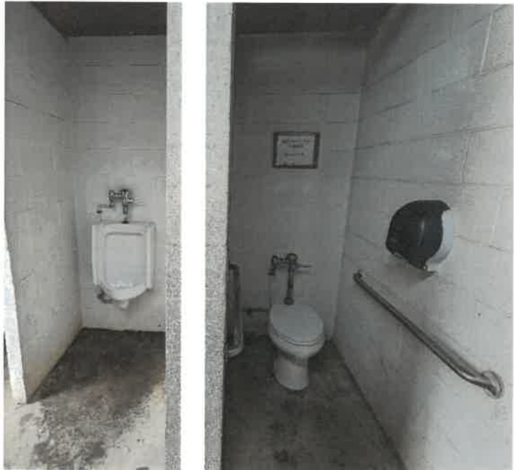
Photos 8 & 9 (above): Urinal and toilet in the interior of the men's restroom
